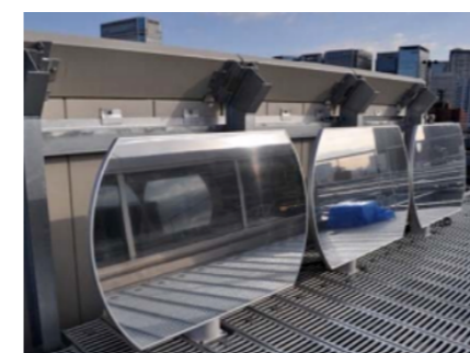
Natural light (solar tracking equipment)
